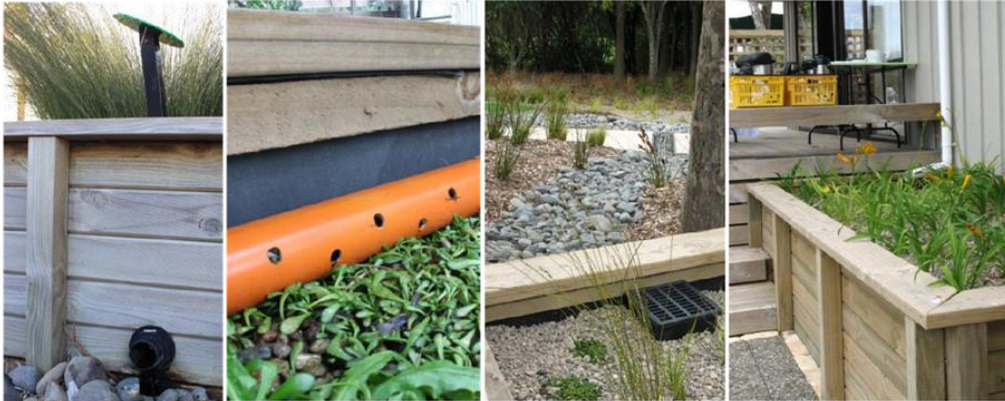
Wooden stormwater planter showing key features from left to right: Outlet of underdrain (to rock-mulched surface swale); a PVC pipe with perforations spreads stormwater evenly, avoids erosion, and is detachable for cleaning; the overflow and black plastic-lining that is waterproof with swale in the background; the wooden box integrated into decking with white inlet downpipe. The plants are oioi ( Apodasmia similis , left), Sellieria radicans (centre), and a perennial, non-native lily (right).
