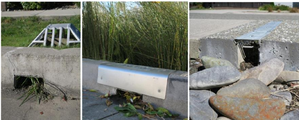
These inlets are too narrow. Centre – an innovative cap allows for stencilling stormwater information but increases risk of blockage. Right – placement of stones reduces potential scour at the bioretention side of the inlet.
