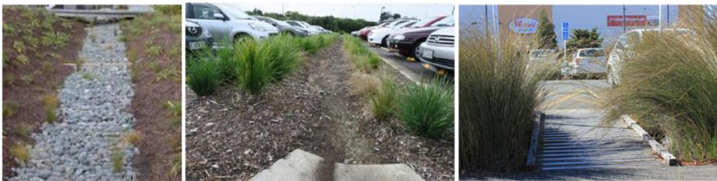
Common faults. Inadequate planting density in swale base and rock mulch that is too big to allow rushes to spread (Left), planting in rows that leave the vital central area bare (centre) and using plants that flop over areas that require clear passage (right). These plants need cutting 2 to 4 times a year so are expensive to maintain.
