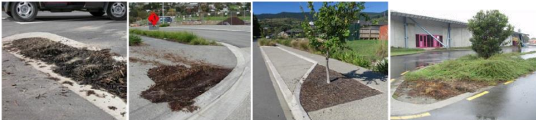
Narrow bioretention and small cell on corners with no protective edges are highly vulnerable to traffic damage
