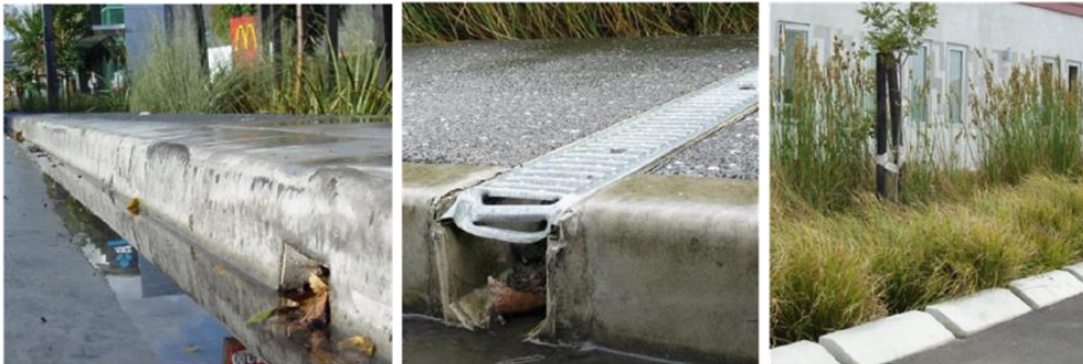
Inlets must be large to avoid being blocked by litter (fast food outlet in left photo) or leaves, especially if deciduous trees are nearby. Plane trees have large leaves and meant the inlets in the centre photo needed at least weekly maintenance. Inlets can be created by having gaps between bricks, but in this case the gap is too narrow (right)
