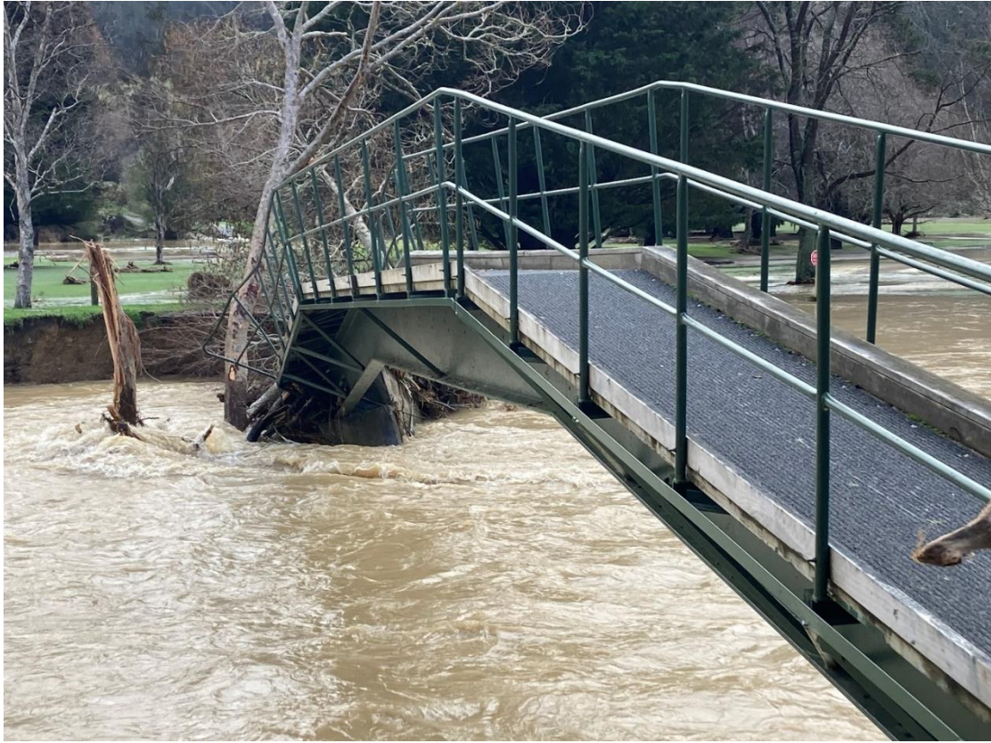
Figure 13: Footbridge at Waahi Taakaro Golf Course damaged beyond repair, August 2022 storm event
