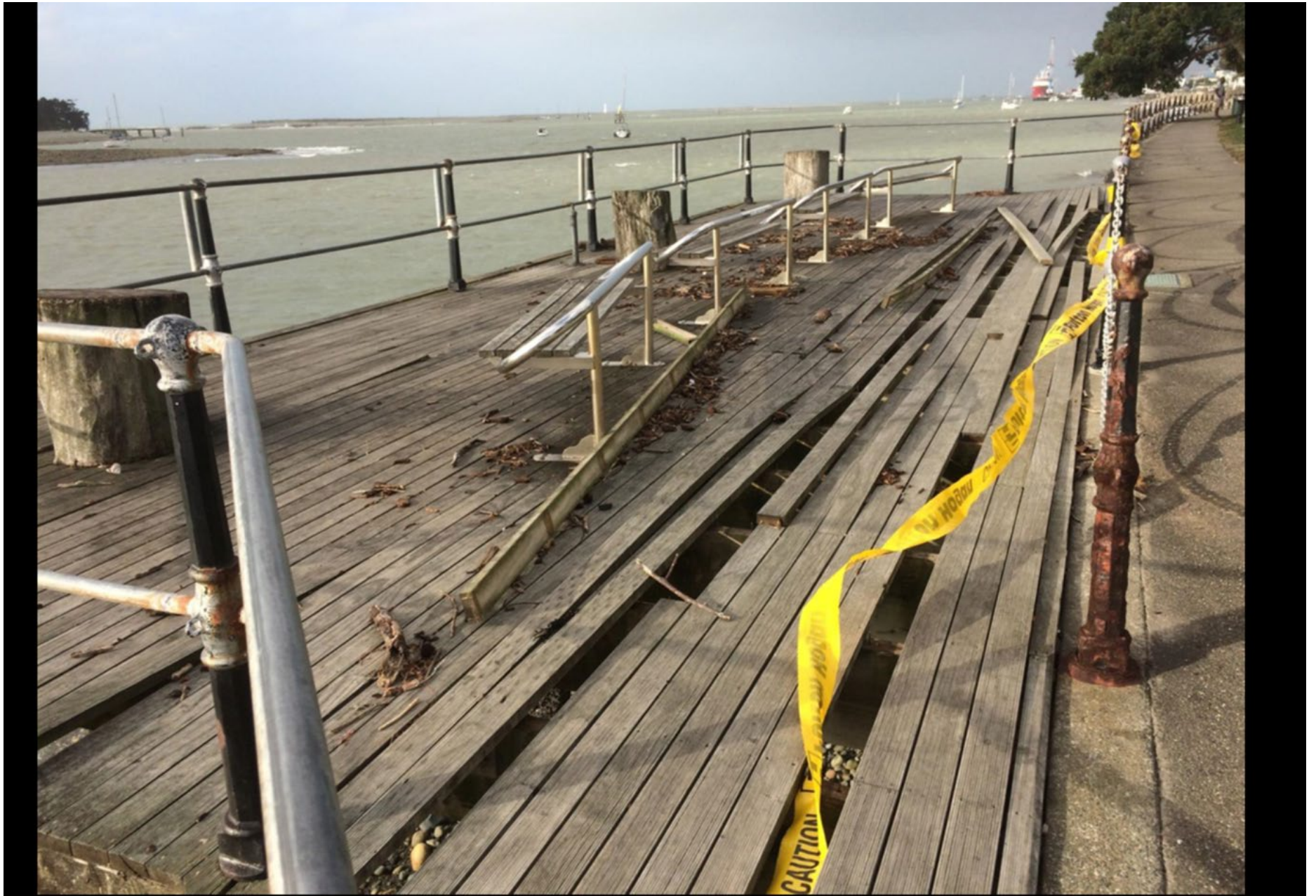
Topside of Fishing Platform after the cyclones
